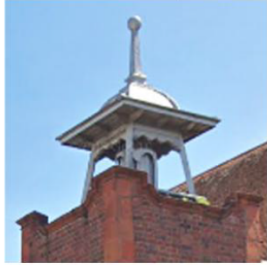
Existing Grovelands Chapel lead covered timber cupola to be refurbished and mounted on flat roof to new tower.
