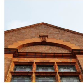
terracotta dressings from arched head of existing western gable Venetian window motif to be reused.
